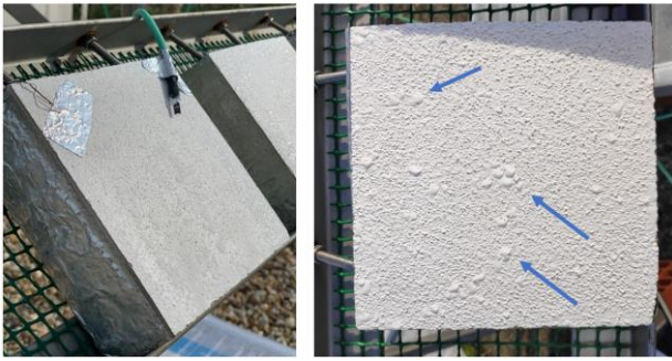
Figure 6: Photographic record of visible surface condensation on specimen S2 of the FCT/UNL roof.
